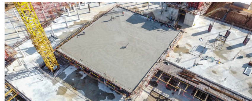
The compatibility of the PERI Systems contributed to the fact that the time and cost framework required for the construction site could be adhered to.
