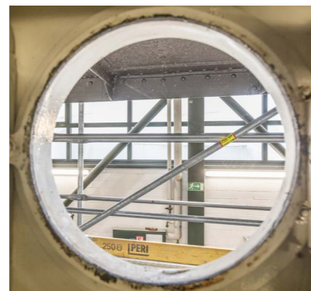
PERI delivered an efficient scaffolding solution to meet the specific requirements of this unique project.
