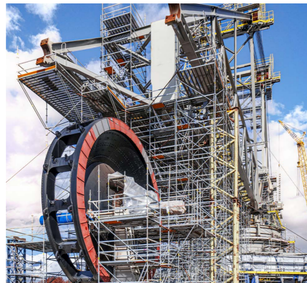
A total of 200 t of scaffolding material was required to scaffold the excavator, a piece of equipment that is over 190 m in length.
