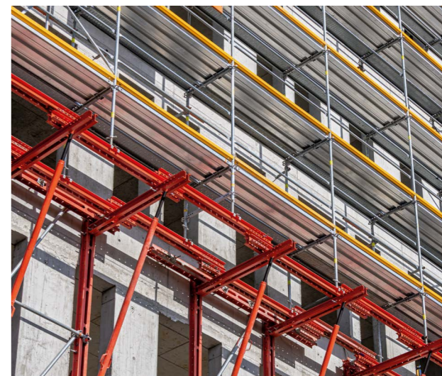
The bracket levels attached to the front are visually and technically outstanding. Ten brackets, each comprising VARIOKIT System Components and installed at a height of approx. 15 m, supported the 10 PERI UP Scaffolding Levels positioned above.
