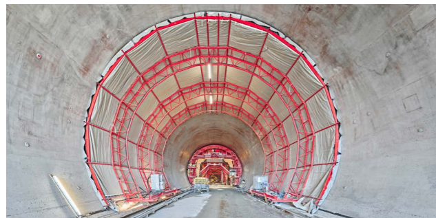
To ensure a high-quality concrete result, the curing gantries controlled the temperature and humidity along the tunnel formwork.
