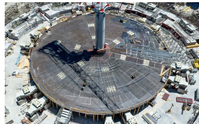
The base in the centre of the ELT was built quickly and flexibly with the aid of MULTIFLEX Girder Slab Formwork.
