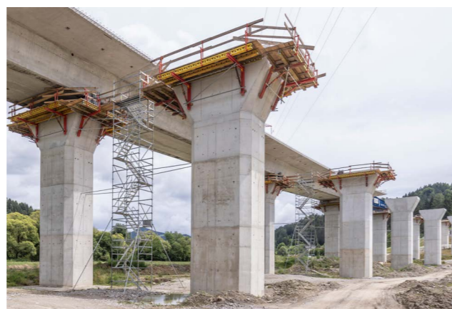
Combined with PERI UP, the flexibility of VARIOKIT made for a safe and fast construction process.
