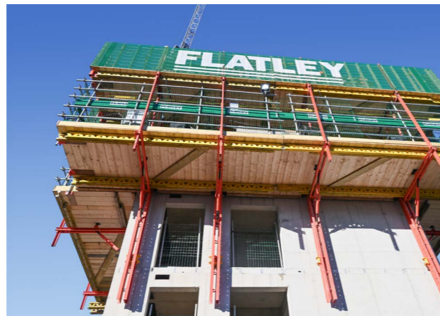
With RCS MAX Rail Climbing Formwork, all platforms could climb simultaneously. This meant that there were no gaps between the platforms, improving worker safety.
