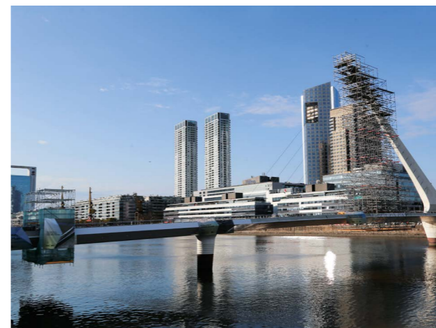
The mobile scaffolding was moved by 3 m every four days, while the sides and underside of the bridge were painted at the same time.
