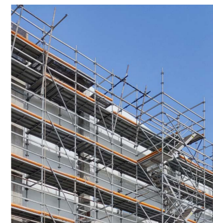
The reinforcement scaffold was later used as a facade scaffold and access solution, which saved materials and optimised the construction site logistics.
