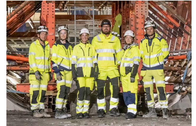
PERI stood ready to advise the customer with their technical expertise and facilitated the progress of the project on site with their know-how and services.
