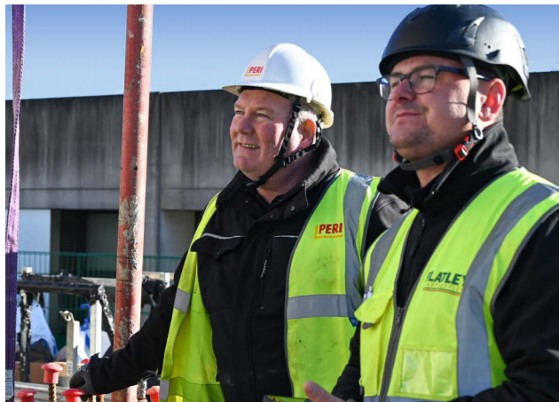
Continuous technical support was an important factor in the success of the project, as was the climbing formwork training that was conducted before initial deployment.
