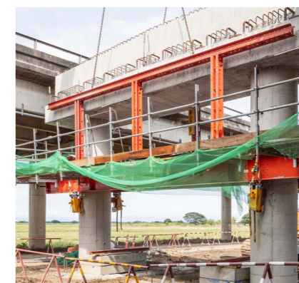
VPS paved the way for short concreting cycles and enabled the 250 cross girders to be completed on time.
