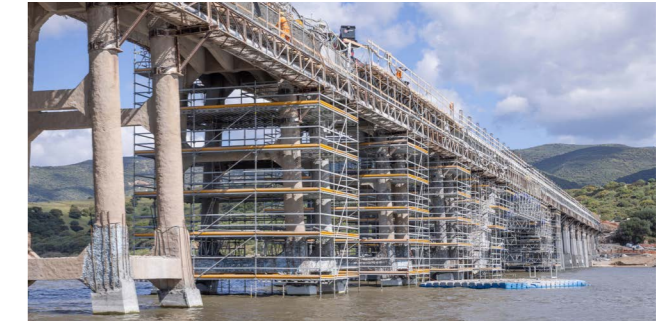
Using formwork and scaffolding systems from a single source accelerated the construction process.
