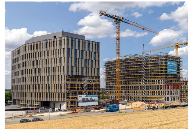
Approximately 5,000 m² of PERI UP Scaffolding was used for each of the individual office towers, which grew upwards during construction and were dismantled again during the installation of the facade.
