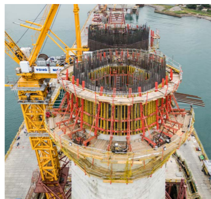
The two PERI SCS and ACS Climbing Systems facilitated quick, safe and efficient construction of the unique pylon structure.
