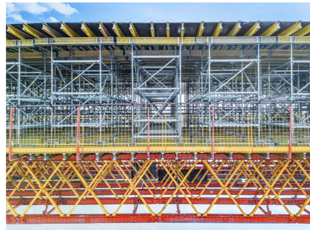
A well-thought-out combination of PERI System Solutions made it possible to construct the spans efficiently.
