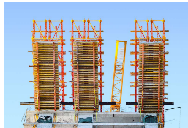
With a cleverly coordinated step-by-step plan, PERI made it possible to construct the sophisticated cantilevered balconies without any issues.
