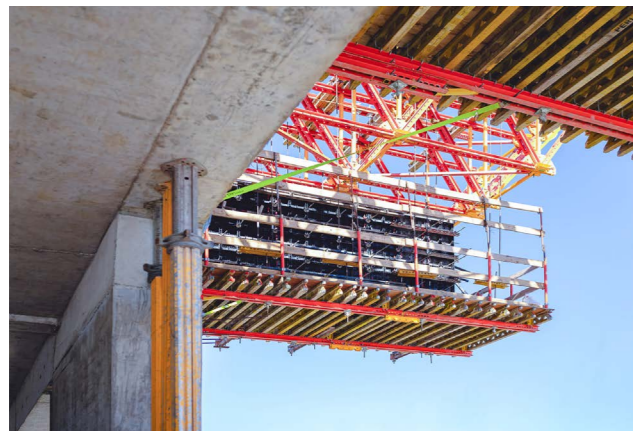
The VARIODECK Steel Waler Slab Tables were very well suited to the project, as these large slab tables facilitated a short concreting cycle.
