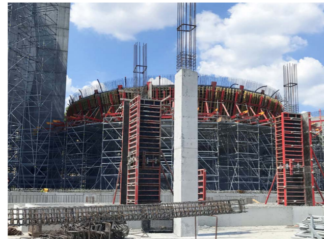
With PERI Formwork and Scaffolding Systems from a single source, it was possible to construct the complex clarification plant in an efficient manner.
