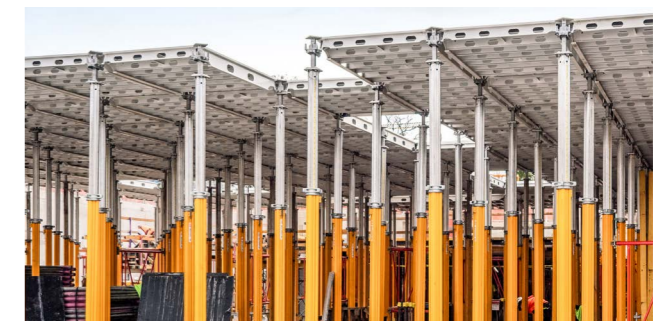
The combined use of ALPHADECK and MULTIPROP saved the customer time and labour.
