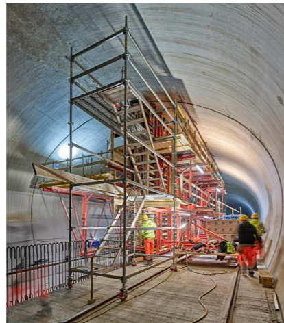
A high level of safety was made possible by the PERI UP Reinforcement Scaffolds when working on the formwork. These are ideal for construction site activities such as reinforcement, forming and concreting.
