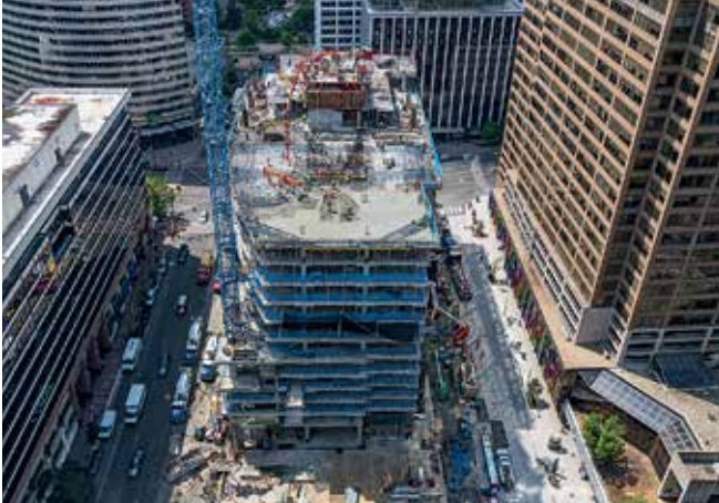
The PERI ACS Core 400 self-climbing formwork shortened the cycle times for the construction of this 31-storey high-rise building.
